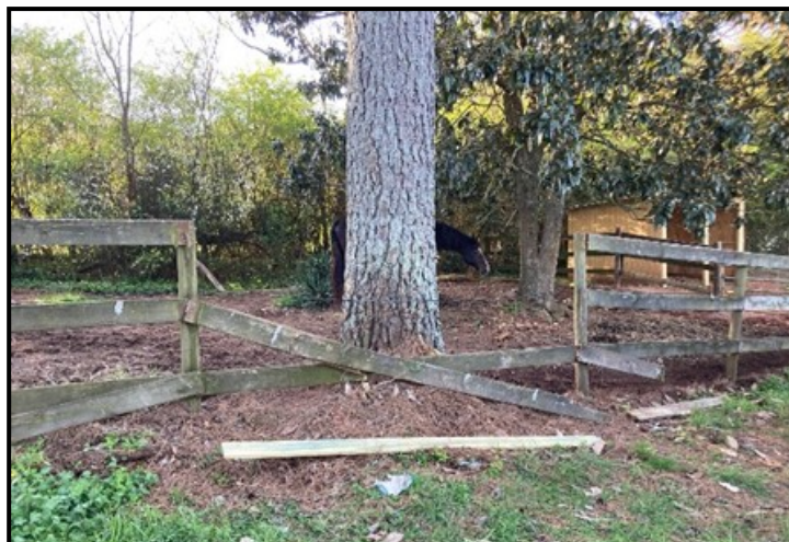
Broken fence boards were a regular occurrence.
